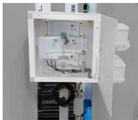
BM sensing panel (includes O 2 , CO, CO 2 monitoring)
